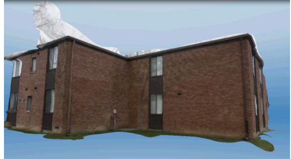
Capture buildings on a cloudy day to avoid harsh window reflections that may distort your model.
